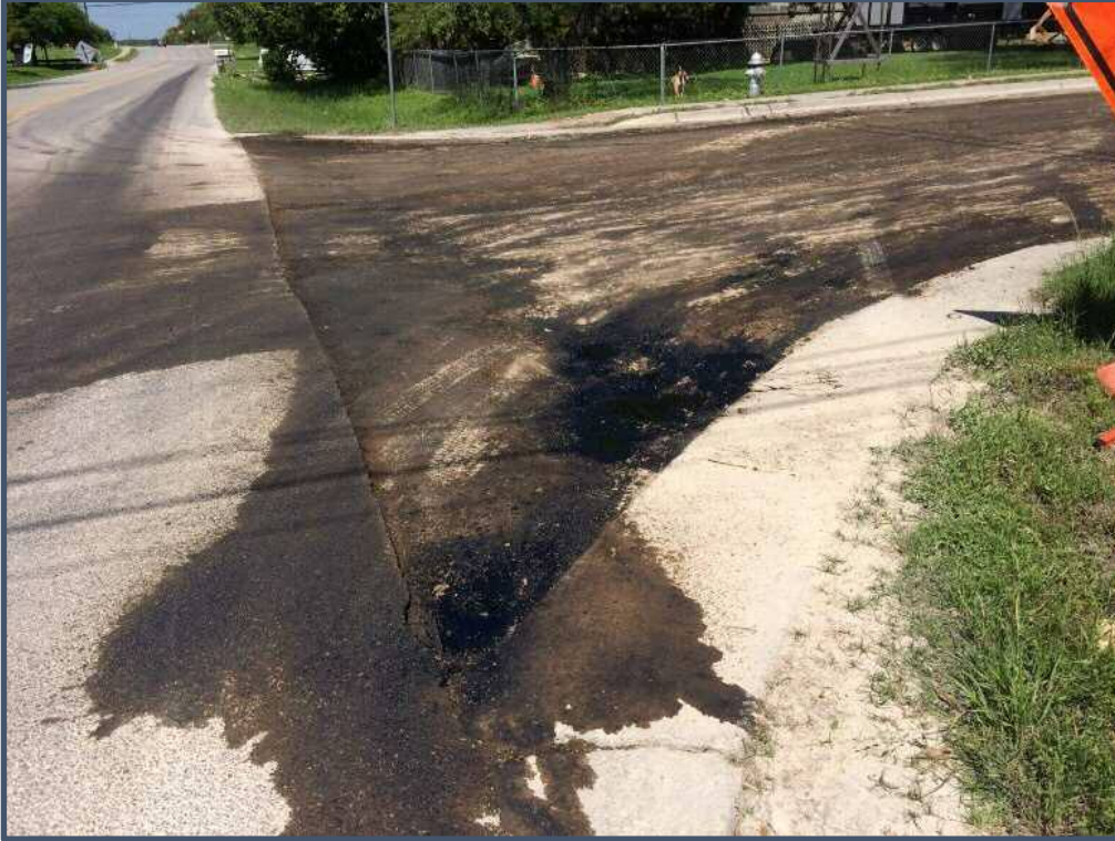
Photo 2: The prepared street after AEP was applied for dust control. Ponding and tracking is an environmental runoff concern.
