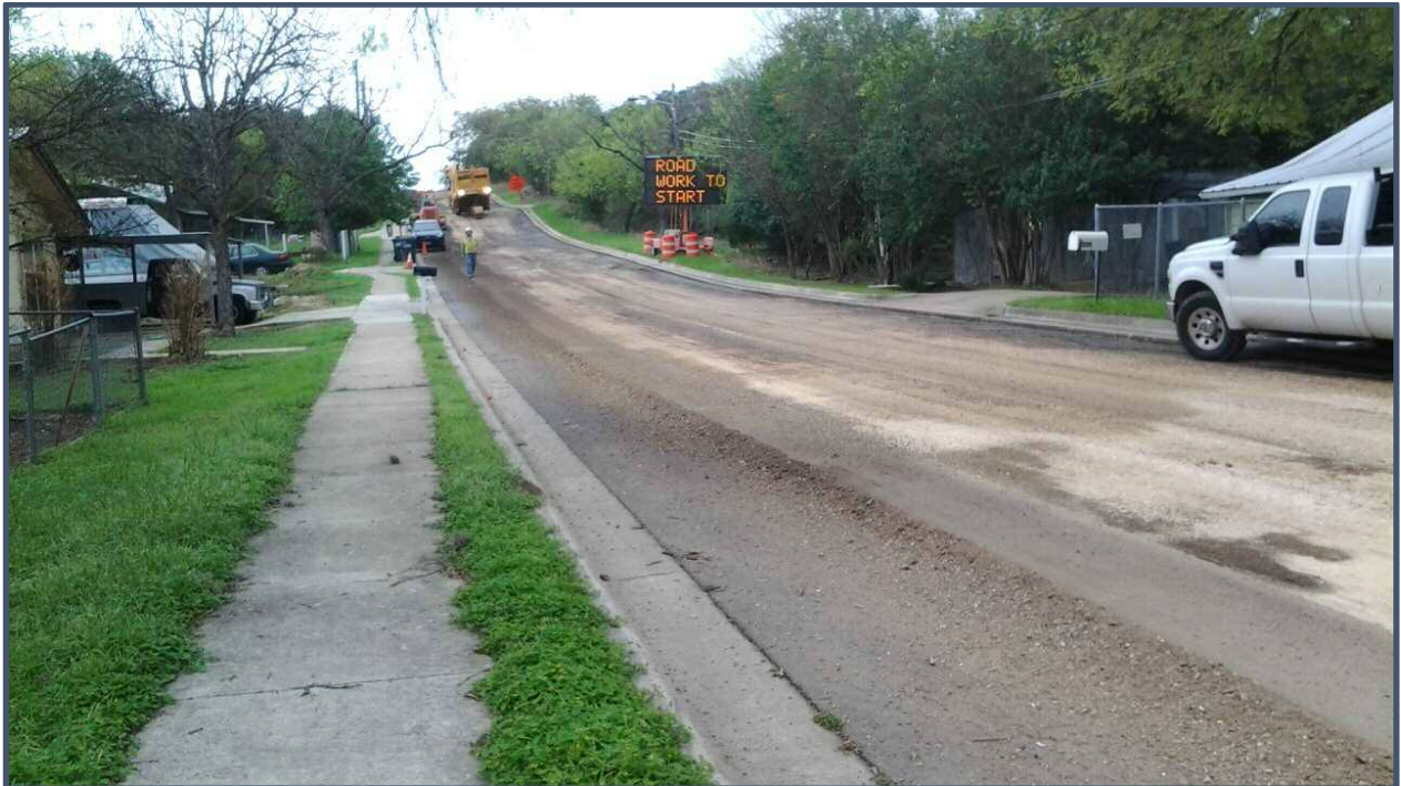
Photo 1: Typical mill and overlay project in San Marcos (2016). Prepared street before AEP oil is applied.
