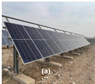
Figure 36.a. Yinchuan PV plant with Trina Solar Vertex (210 mm) monofacial configuration
