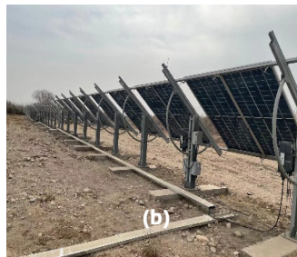
Figure 36.b. Yinchuan PV plant with Trina Solar Vertex (210 mm) bifacial configuration
