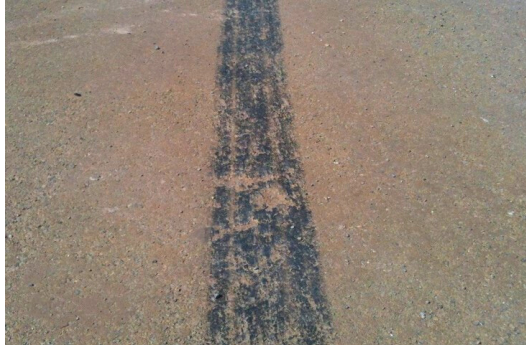
TSW after 24 hours of curing – close up Skid marks only leaving a black mark on the surface.
