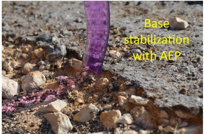
AEP Prime coat in Florence, Texas: Less than 1 inch penetration
